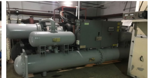
Solids Workshop Double Head Screw Chiller
