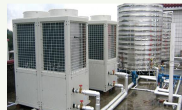
Air source pumps
