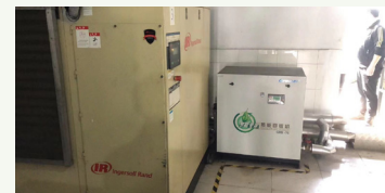
Waste heat recycling by an air compressor
