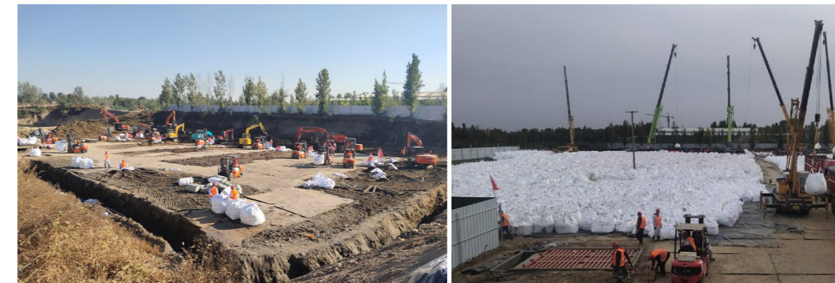
紅樹林鋁灰鋼渣處置現場 BBMG Mangrove's aluminium ash and steel slag disposal site
