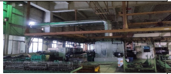
Paint spray booth and exhaust piping after rectification
