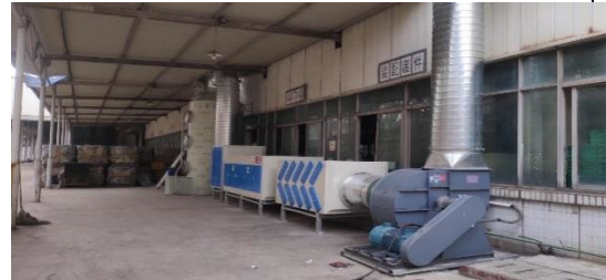
Paint spray waste gas treatment facilities
