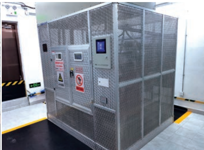
▲ Dry type transformer
