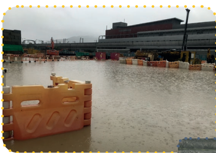
Typhoon-caused flooding on construction sites
