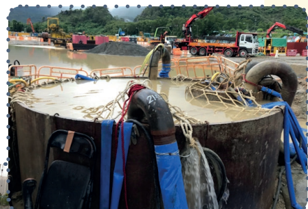
Water storage tank overflow
