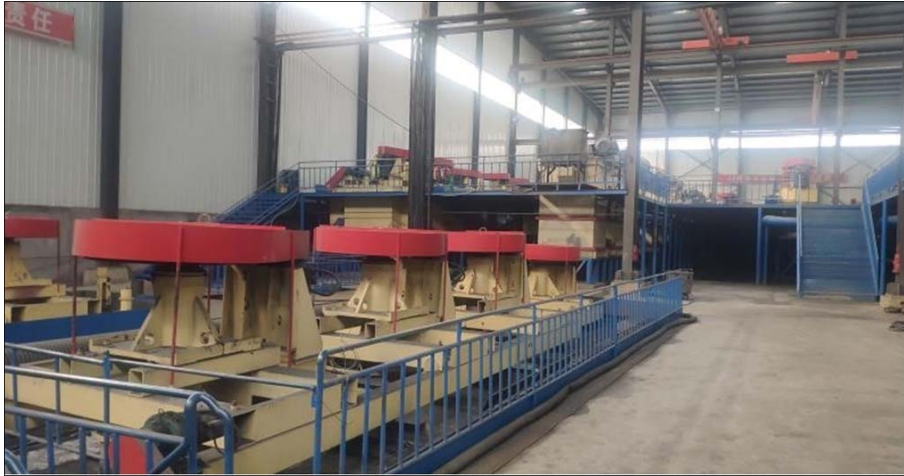
Figure 8–6: New flotation machines
