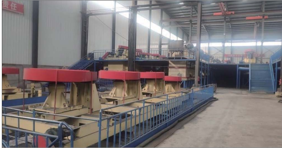
Figure 8–6: New flotation machines
