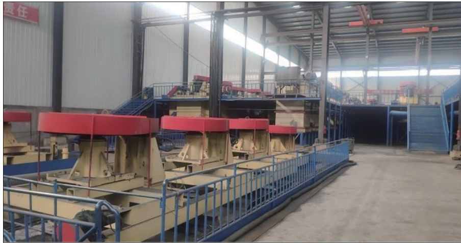
Figure 8–6: New flotation machines
