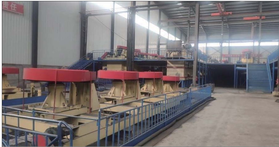
Figure 8–6: New flotation machines
