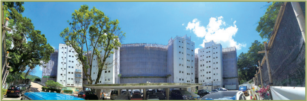
Renovation works at Carolina Gardens, The Peak 山頂嘉樂園之翻新工程
