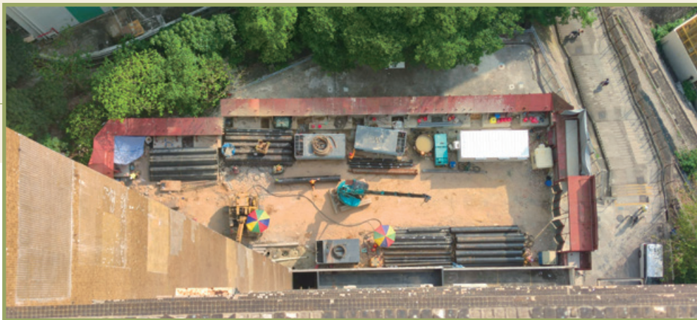
Industrial redevelopment at No. 22 Yip Shing Street, Kwai Chung 葵涌業成街22號之工業重建項目
