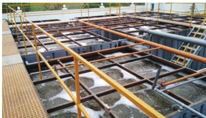
Sewage Treatment Facility in Vietnam Factories 越南廠區污水處理設施
