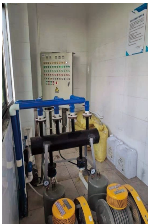
Hainan food factory - Wastewater treatment facility
