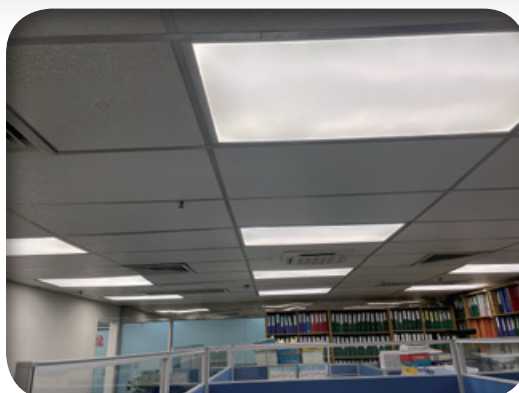
Energy saving lightings (LED lightings) are installed in our office
