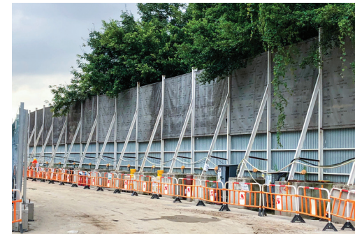
A six-metre high noise barrier was erected along the site's boundary to further minimize construction noise
