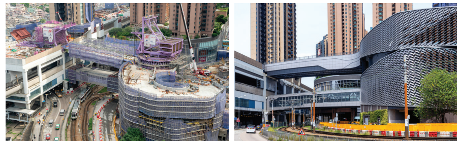
The first-ever rotational bridge launching construction at The YOHO Hub is expected to be operated in 2023
