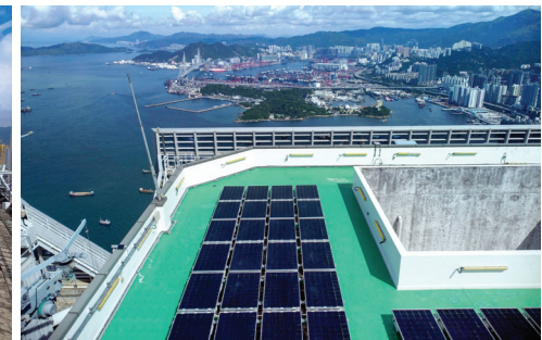
Solar panels in ICC
