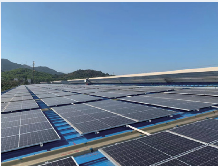
Solar panels on the rooftop of a production plant 生產廠房屋頂的光伏發電設備
