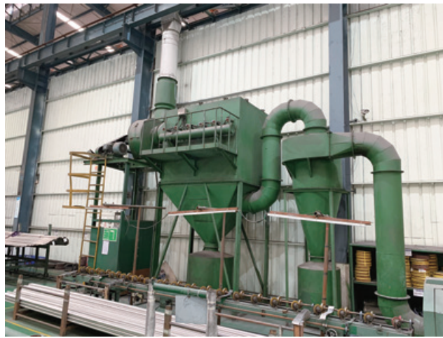
Production plants equipped with dust collectors with filter bags 生產廠房中設有布袋除塵器
