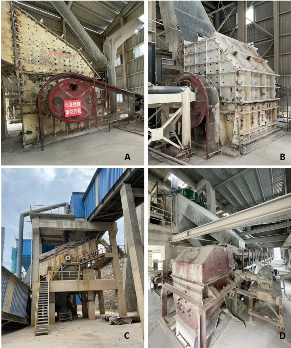
Figure 8-3: Phase I processing plant
