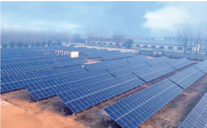
The PV Power Generation Subproject for Megawatt Water Electrolysis Hydrogen Production
