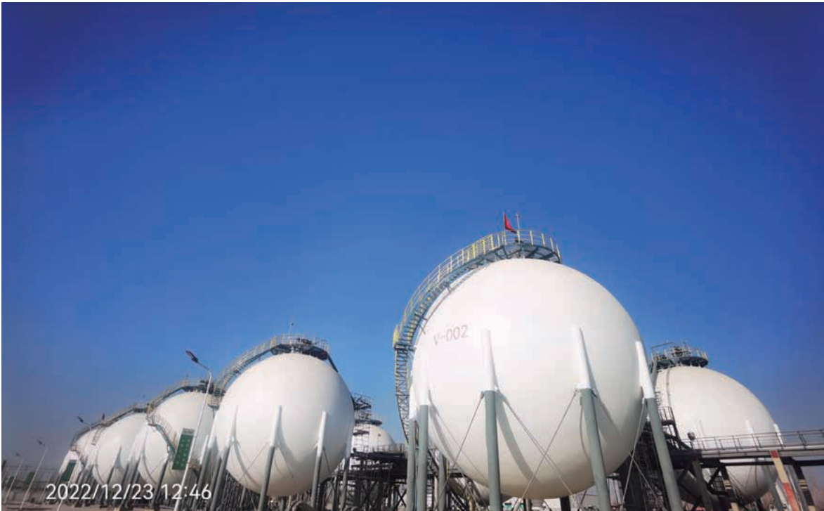
Hydrogen balloon tanks of the green hydrogen demonstration project
