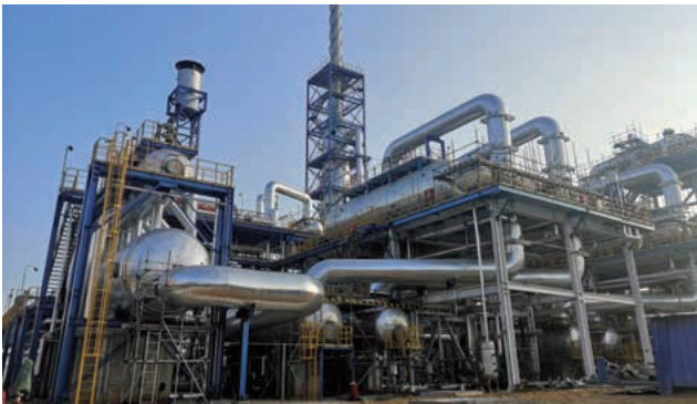
The 180 KT/a sulphur recovery unit with low emission sulphur recovery engineering design technology at Fujian Refining & Ethylene Project (FREP)
