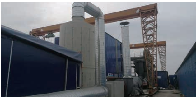
VOCs treatment facility of Shenghong Petrochemical Engineering Project Department of Sinopec Tenth Construction Co., Ltd.
