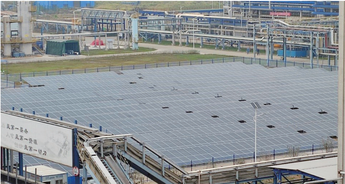
PV Power Generation Project of Sinopec Catalyst Co., Ltd.
