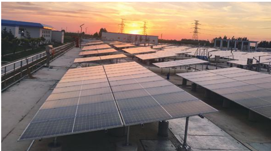
In-plant solar photovoltaic facilities in Zibo Waste Water Treatment Project (Plant 1) 淄博污水處理項目(一廠)的廠內光伏發電設施
