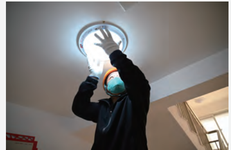
▲ Investigation and rectification of potential fire hazards in the offices
