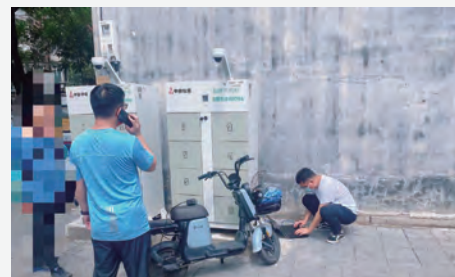
▲ Charging piles help residents charge safely
