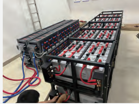
▲ Power backup site of Guangxi telecom communication shelters with power supply facilities supporting
