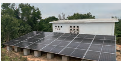
▲ Solar panel and machine room
