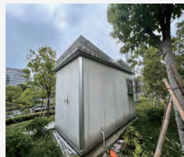
▲ The energy storage equipment in the station and photovoltaic equipment on the top of the station
