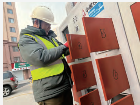
▲ Investigation and rectification of hidden dangers of energy battery exchange cabinets
