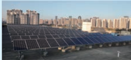
Photovoltaic Power Generation System in Hefei Capital Outlets
