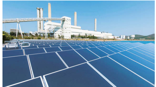
■ A 1.1-MW solar power system is installed at Lamma Power Station.
