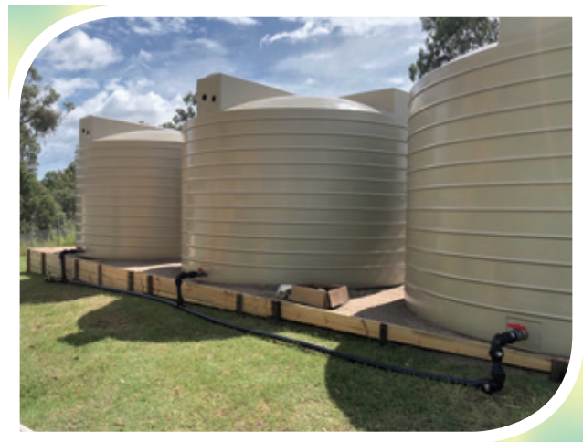
The application of reverse osmosis treatment technology at Accensi to treat contaminated storm water for reuse in our products has allowed us to replace the use of town water and conserve precious resources.
