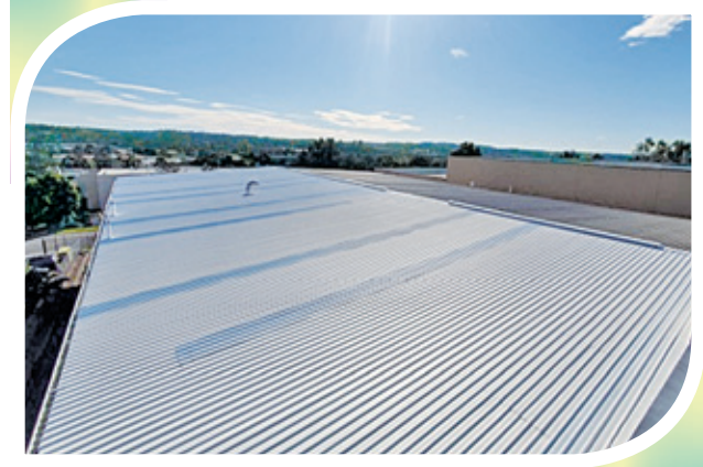
The application of heat reflective paint (SkyCool) on the roof helps keep Lipa’s warehouse cool and reduces energy consumption.
