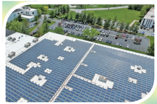
Solar panels are installed at Vitaquest’s headquarters to generate electricity onsite and hence reduce purchased electricity.
