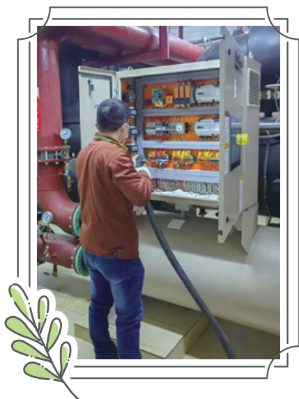
Inspection of high-low voltage power distribution equipment in Parkson Mianyang store 百盛綿陽門店高低壓配電設備巡檢
