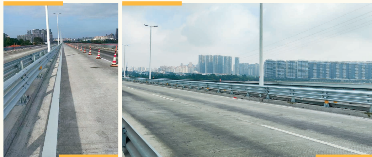
Shantou Bay Bridge has upgraded its corrugated beam barriers to three-beam safety barriers for better collision protection and safety.
