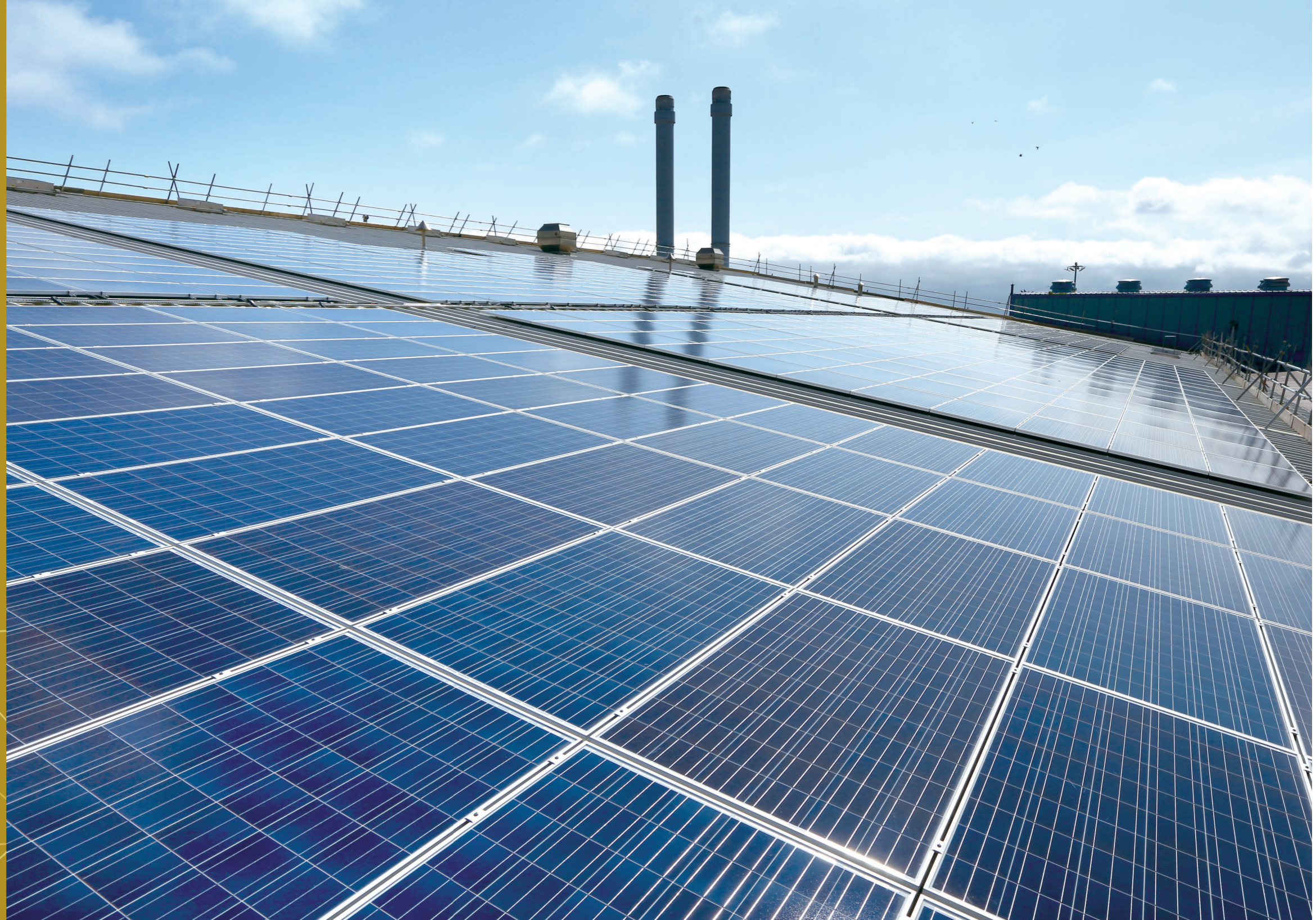
Northumbrian Water - Solar panels installed at Bran Sands Sewage Treatment Works, Teesside, supporting its ambitious goal to be net zero by 2027.
