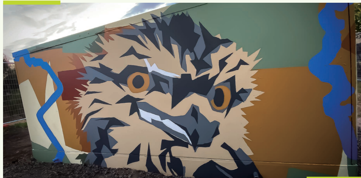
VPN participated in Victorian Government's Neighbourhood Battery Program Initiative, installing a battery system in Tarneit to store excess solar power and improve energy reliability for up to 170 homes.
