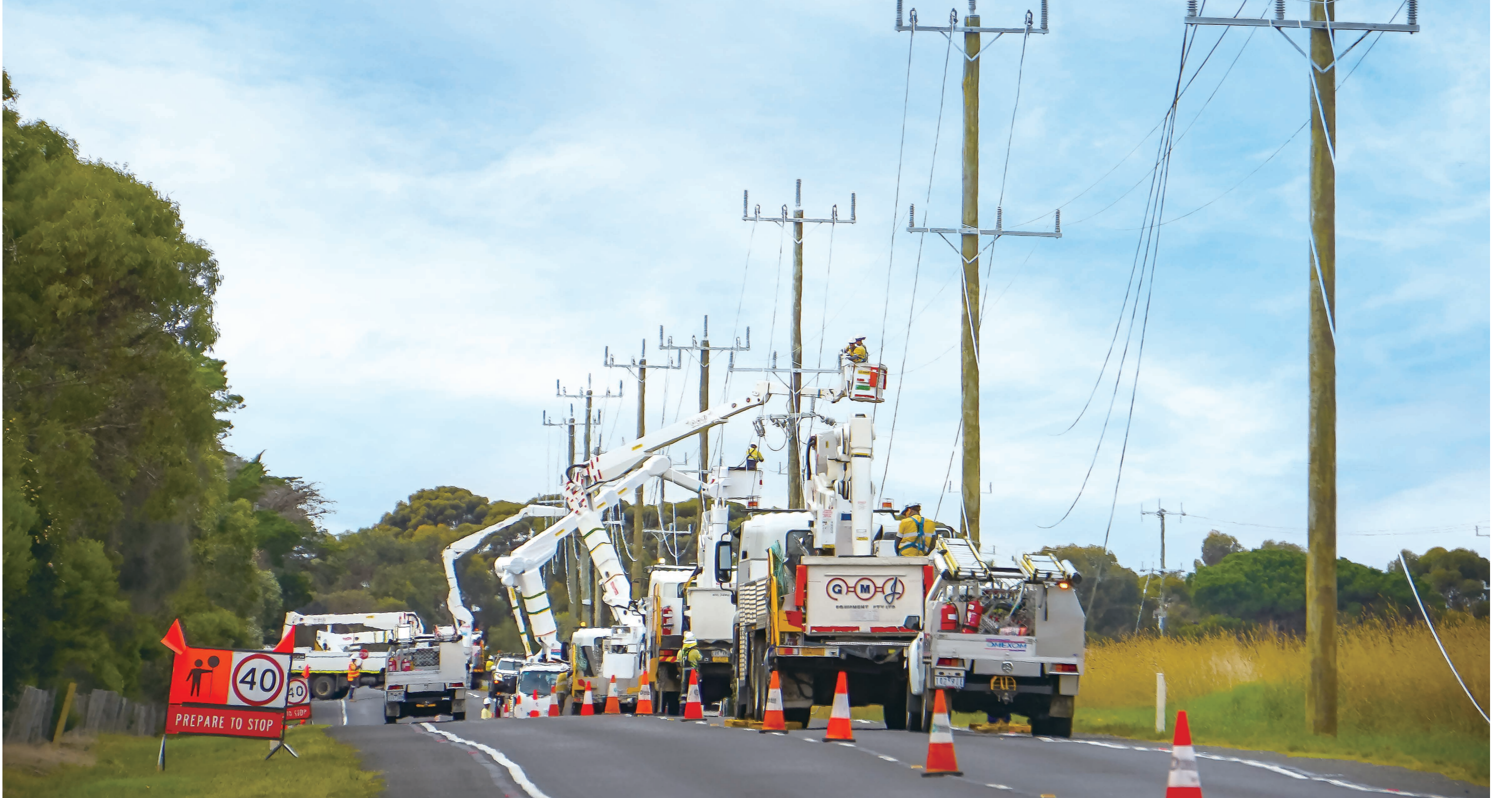
Victoria Power Networks field teams upgrade overhead powerlines to reduce bushfire risk in Western Victoria, Australia.
