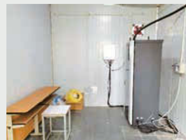
Waste gas emission monitoring station room
