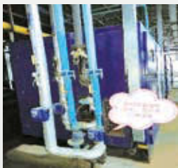
Air compressor residual heat recovery unit
