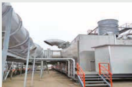
Installation of "zeolite rotor + RTO"
