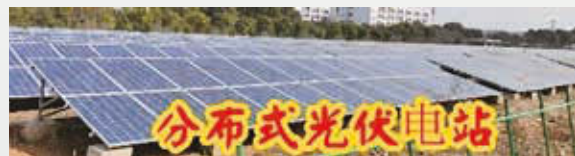
Distributed photovoltaic power plant
