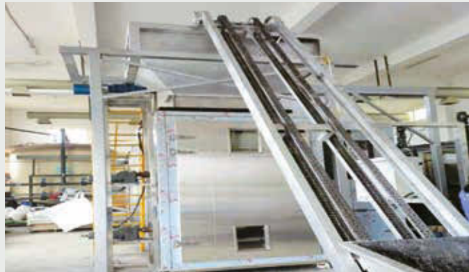
Sludge drying device
