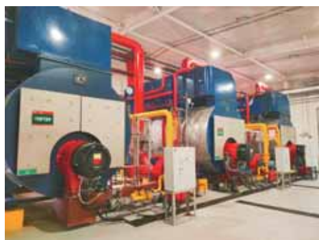
靖宇工廠天然氣鍋爐 Natural Gas Boilers in Jilin Jingyu Factory
