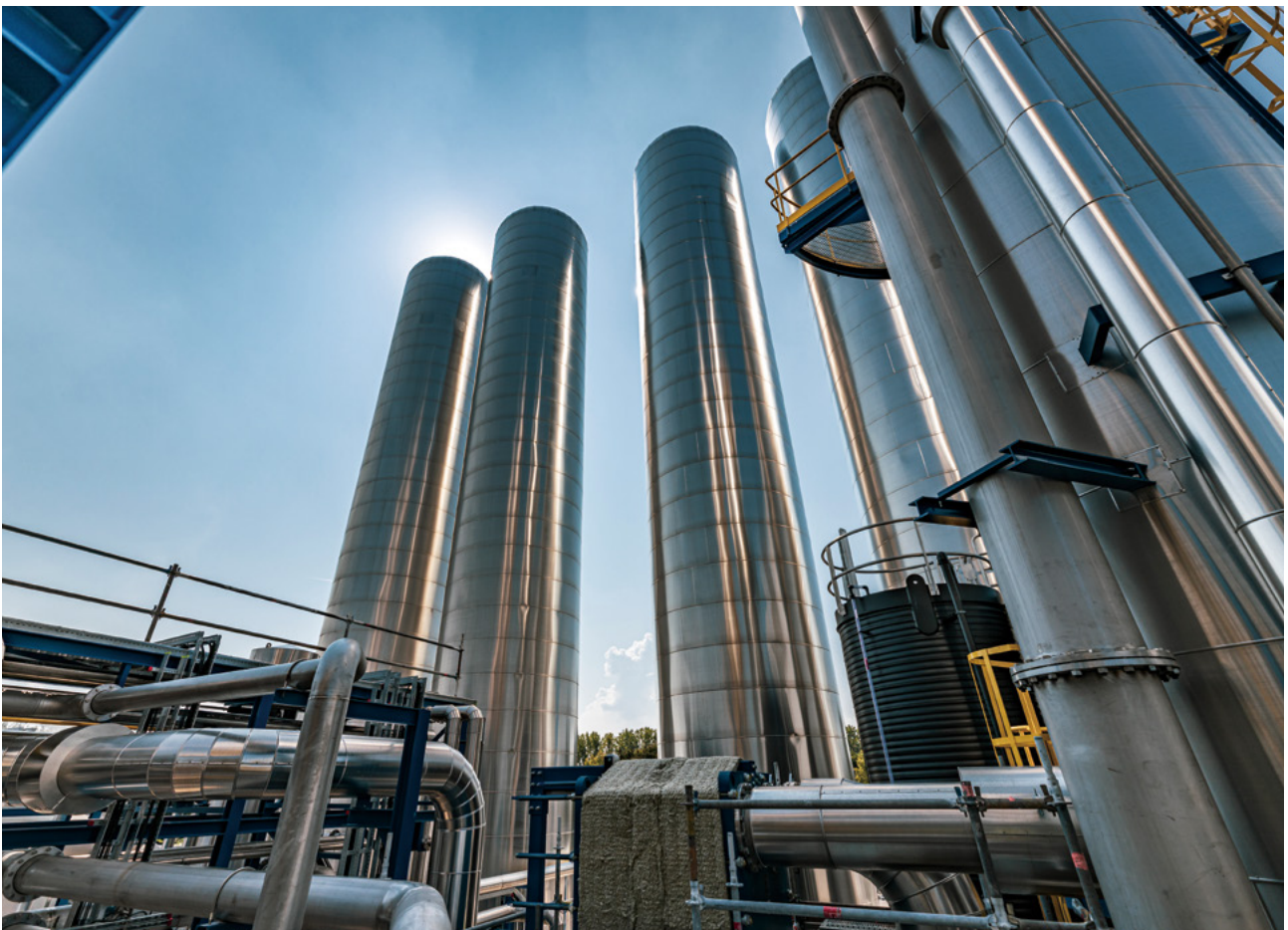
AVR's CO 2 capture plant in Duiven
