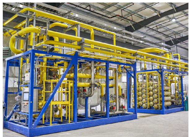
EDL's Wood Road RNG Facility in Michigan
