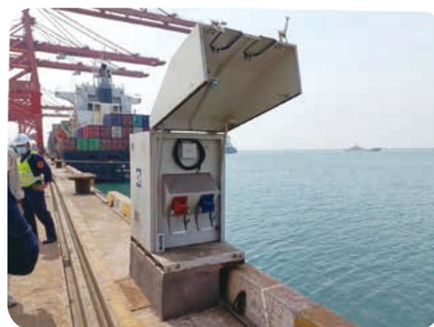
Lianyungang New Oriental Terminal completed the construction of two sets of 5MVA high-voltage shore power supply systems and supporting shore power socket boxes, and upgraded five sets of low-voltage shore power boxes to meet the needs of shore power connections for various vessels.
