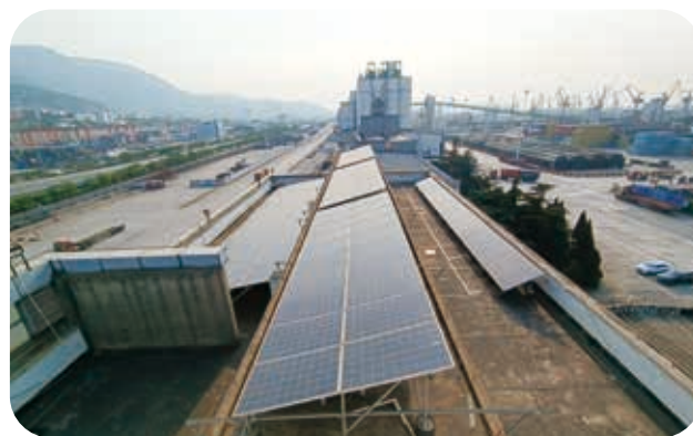
Lianyungang New Oriental Terminal has installed a distributed photovoltaic grid-connected power generation system on the roof of its office building, with an installed capacity of 100kWp and an annual power generation of 110,000 kWh.
