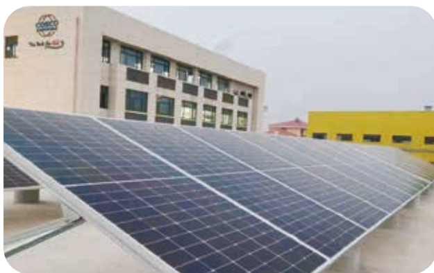
CSP Wuhan Terminal has installed 1,063 pieces of 545WP monocrystalline silicon solar photovoltaic modules on the roof of 5,768 square meters in the port area, with a designed capacity of 0.578MWP, providing clean power for the production in the port.
