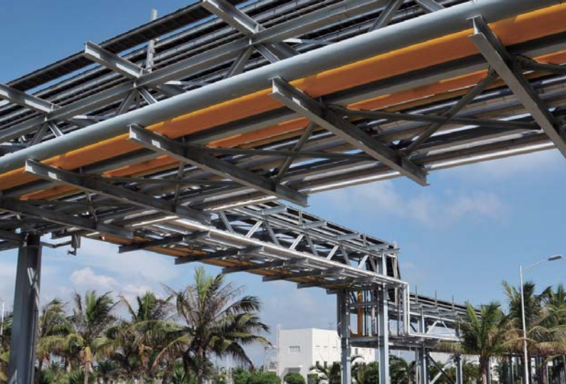
➤ Hainan Phase I methanol plant pipe rack
