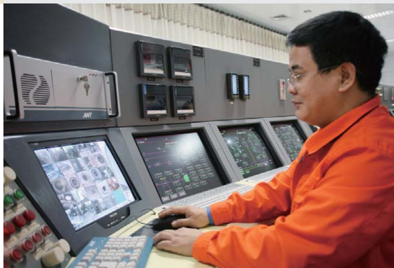
➤ The operator of the main control room is carrying out routine inspection
