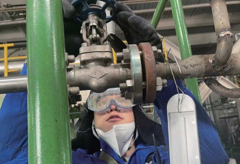
Adjusting refill valve of ammonia pump tank
