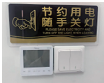
Electricity saving notice at office
