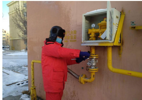
Equipment maintenance under cold wave weather
