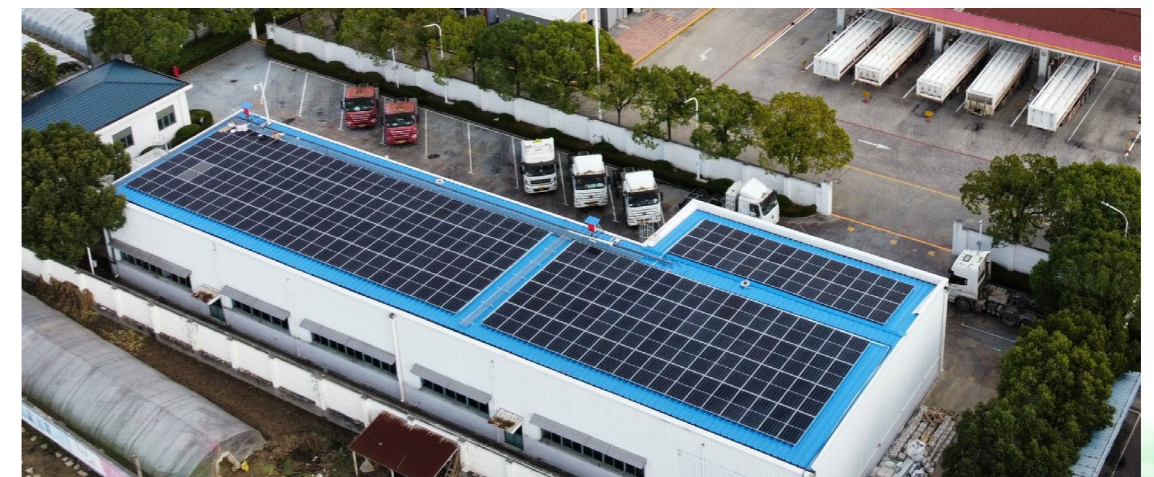
The rooftop photovoltaic project at the Kunlun Energy Shanghai CNG station
