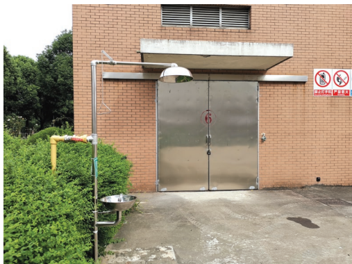
Operation area equipped with eye washers
