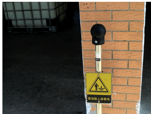
Production area equipped with electrostatic removal device
