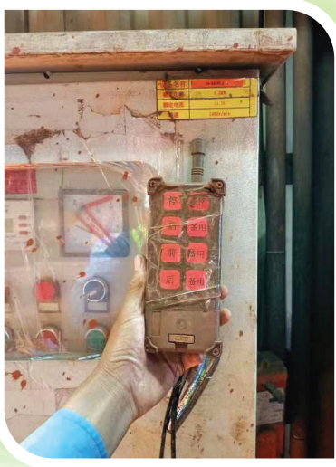
Interlocking Device Controllers
