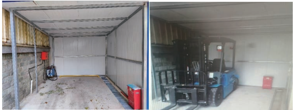
Special Charging Piles for Lithium Battery Forklifts to Prevent Fires Caused by Lithium Battery Charging Built by Subsidiaries
