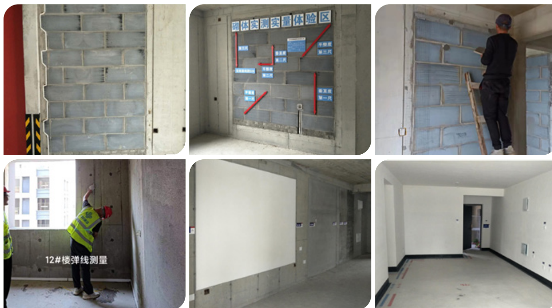
Thin plastering system of Anyang Jianye City
