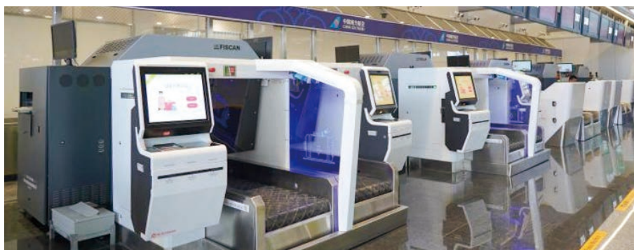
Self-service baggage check-in machines 自助行李托運設備
