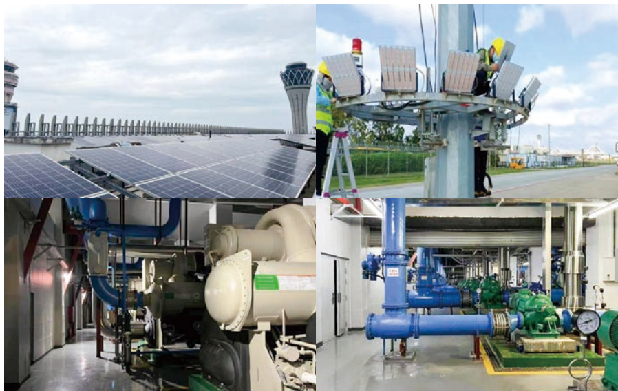
Energy conservation and emission reduction project in Meilan Airport 美蘭機場節能減排項目
