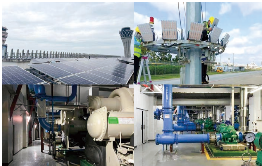
Energy conservation and emission reduction project in Meilan Airport 美蘭機場節能減排項目
