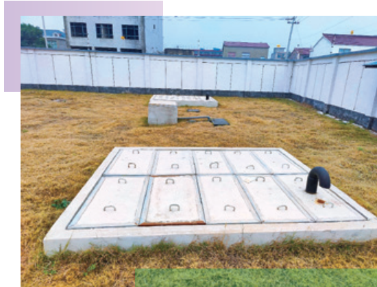
Sewage Discharge Facilities at Anhui Huoqiu Huayang Power Plant 安徽霍邱華陽電站排污設施
