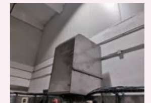
Equipment is installed with sound enclosure
