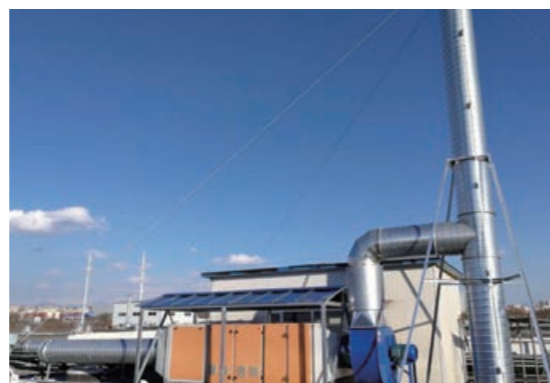
VOCs treatment facility
