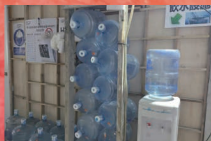
Providing drinking water at the construction site 在施工現場提供飲用水
