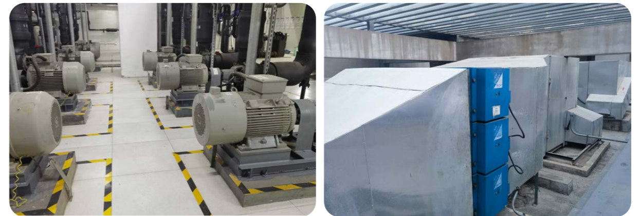
After an energy-conservation upgrade with inverter technology, the air conditioning pumps and exhaust fans at Qingdao Jinmao Harbour Shopping Centre save approximately 20,000 kWh of electricity in a year.
