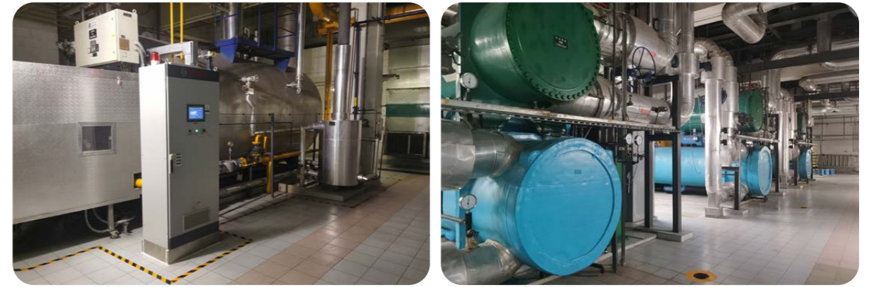
Jinmao Tower's HVAC system equipment
