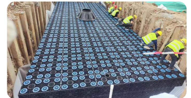
Construction site of the addition of rainwater modular cisterns at Foshan Chao'an Jinmao Residence
