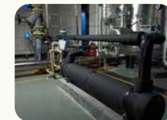
Laundry Hot Water Recovery
