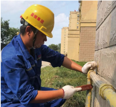
Photo: Outdoor Riser Maintenance
