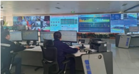
Centralized control room of Sixth Company of QHD Port
