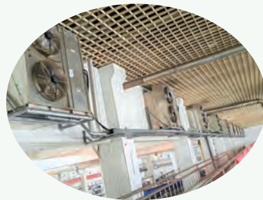
The heat pumps of Tsingtao Brewery's No. 5 Brewery
