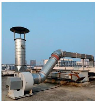
Waste gas treatment facility 廢氣處理設施
