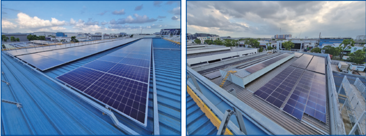
The rooftop solar systems
