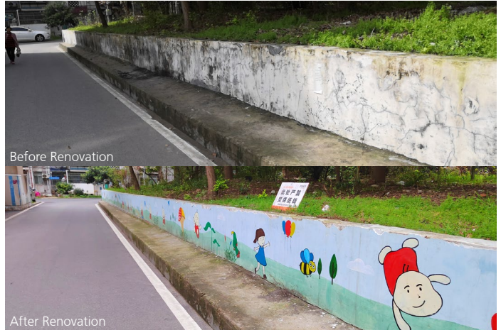
The Low Wall of Gangyuan New Village was Revitalized by Fun Painting to Reduce Fire Hazards
