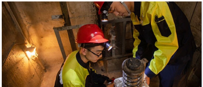
Vanke Service Maintenance Personnel Performed the Fine Adjustment and Maintenance of the Elevator Pit
