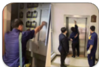
Outage and lock ladder ladder 斷電、鎖梯
